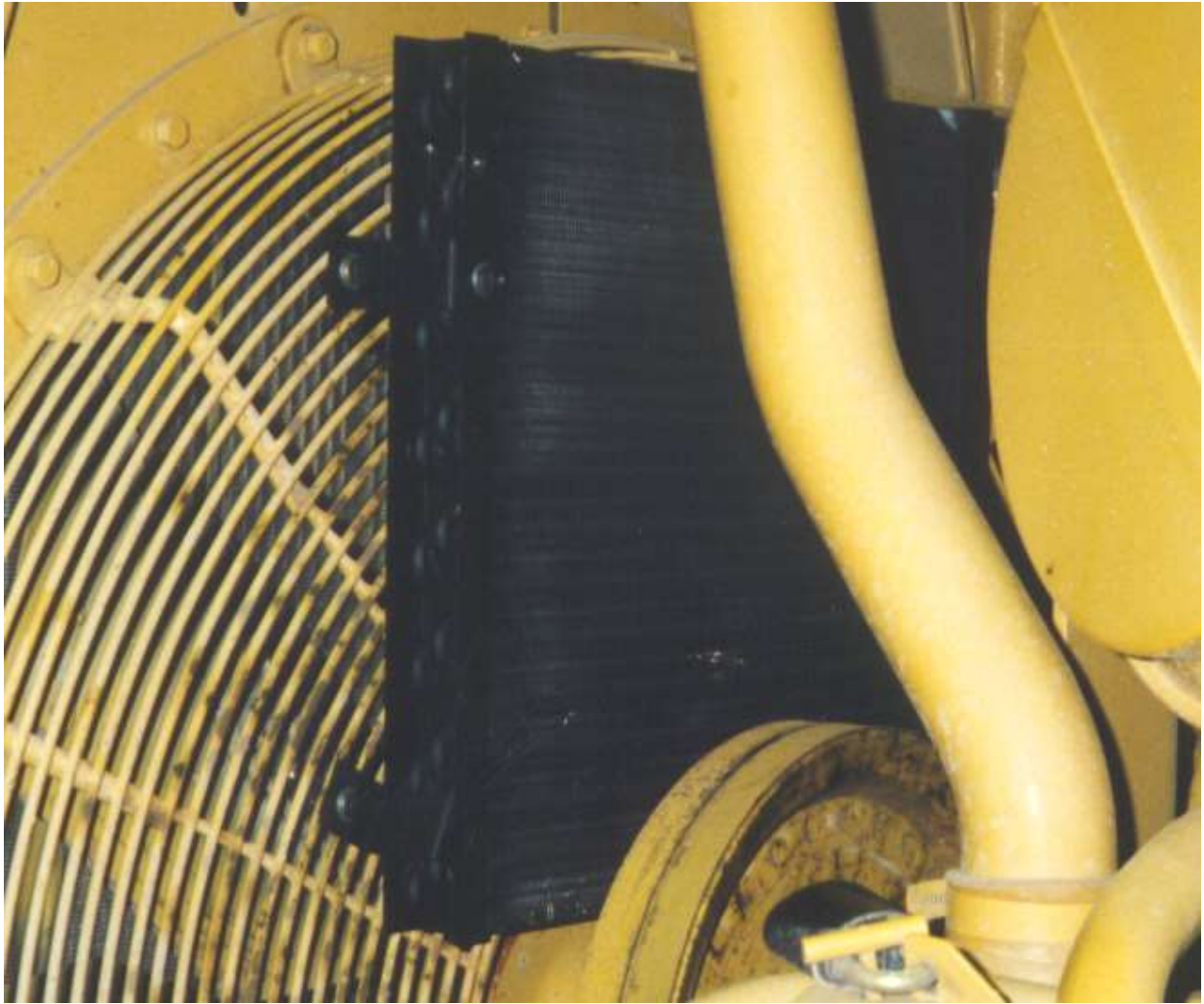
Left side of the condenser with hold down brackets in place.
