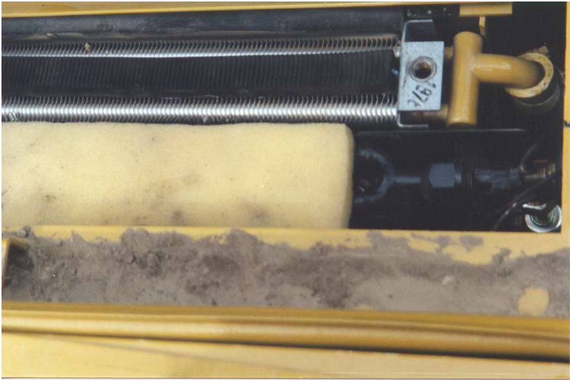
Top of evaporator assembly in heater box.
